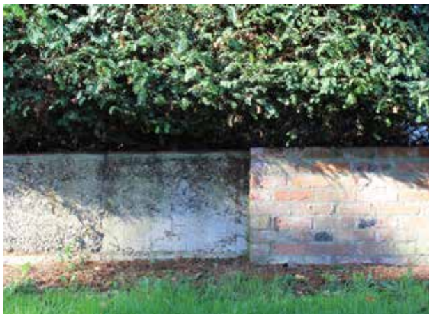
Figure 82: Replacement of low brick wall with concrete, which is out of keeping with the material palette of the area
